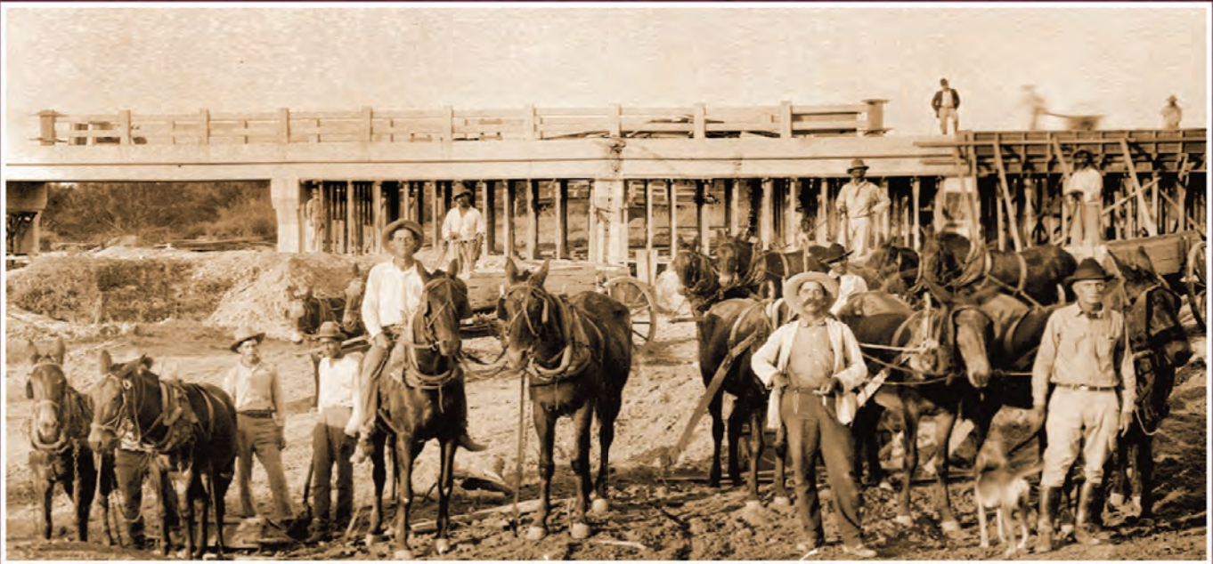
Highway bridge construction site, Webb County, Texas, 1924 — The first job for founder H.B. Zachry, '22 and the start of a company that would later lead the domestic engineering, construction and maintenance industry.
